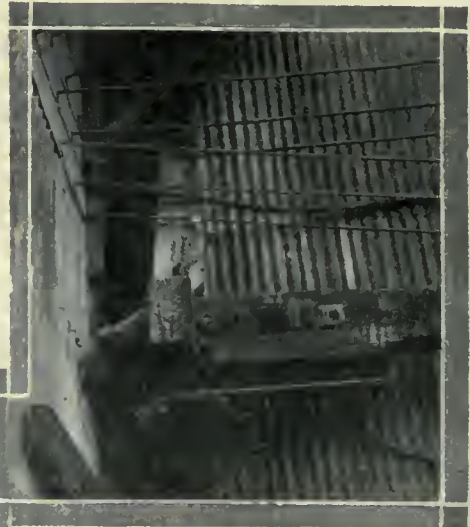
FIG. 2. TOP OF BRACE SHOWN IN OPPOSITE PICTURE, WITH METHOD OF BRINGING PRESSURE ON BLOCKS BY CLAMP-BOLT.
